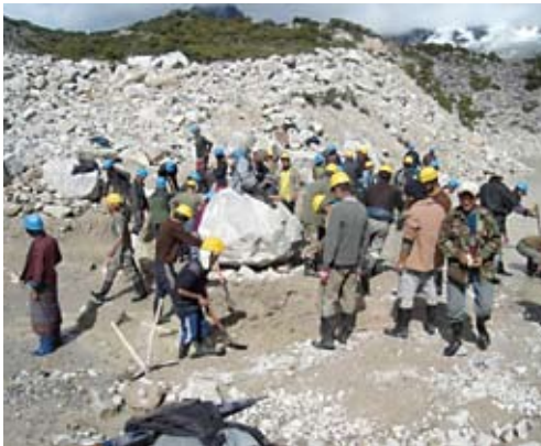
Photo. 10 GLOF hazard mitigation works in Thorthormi Tsho, Lunana. Photo taken by Mr. Karma Toeb (DGM).
